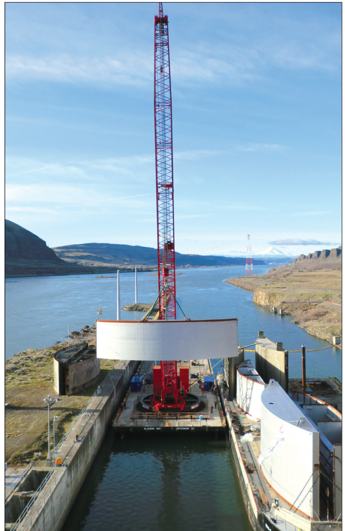
Advanced American Construction replaced the mechanical drive system at the John Day Lock and Dam.
